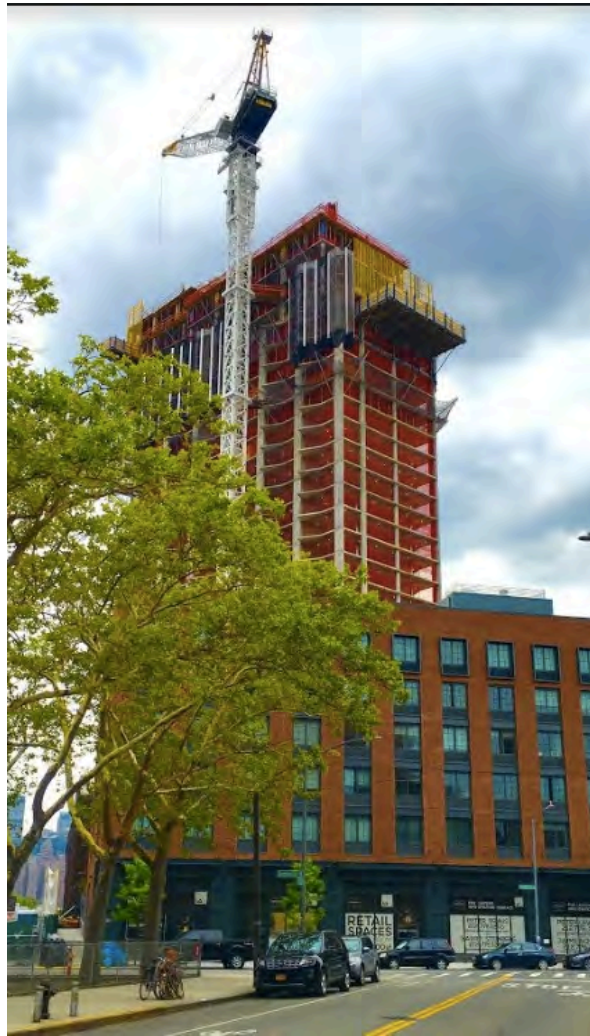
This tower is 37 Blue Slip, which is part of the Greenpoint Landing mega-development.
